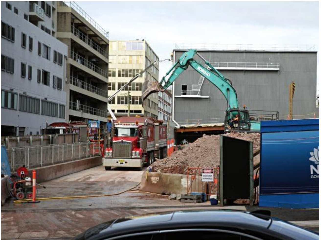
Work is under way at the Crows Nest Metro site. Picture: Adam Yip
